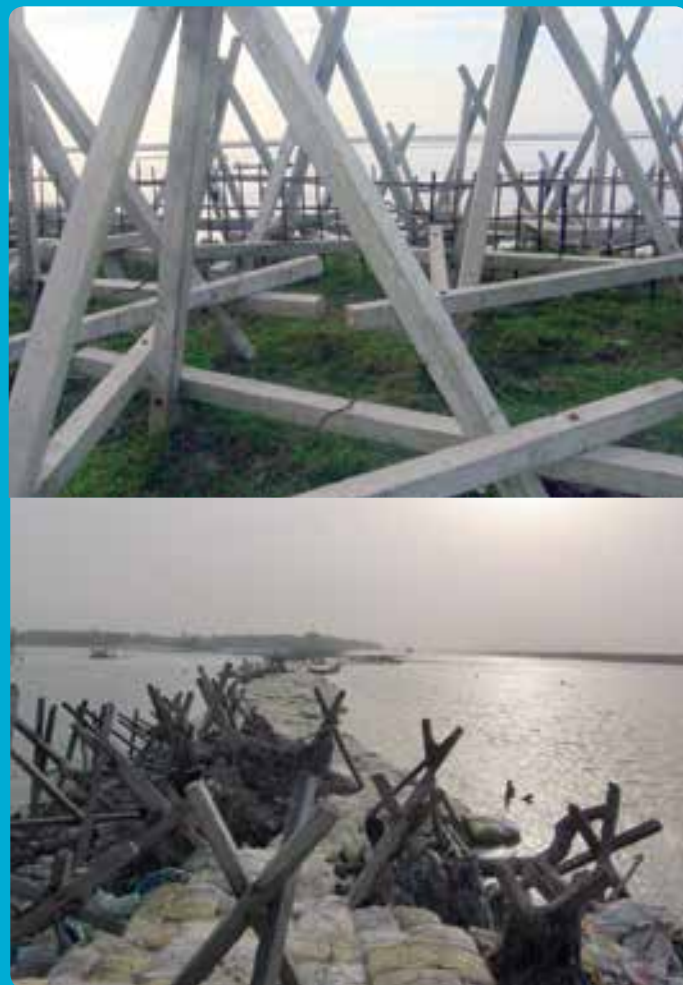
Figure 51: RCC porcupines along a river bank (top) and combined with sandbags to form a bar projecting into the Koshi river (bottom)
