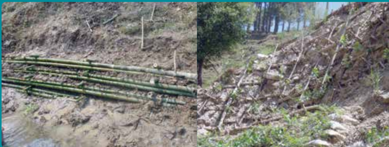
Figure 16: Newly constructed live crib wall made of bamboo (left) and live crib wall on a slope (right)
